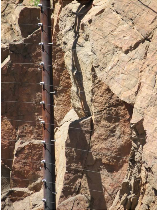
Figure 3.13. Close-up of Rockfall Alarm Fence in Byers Canyon
