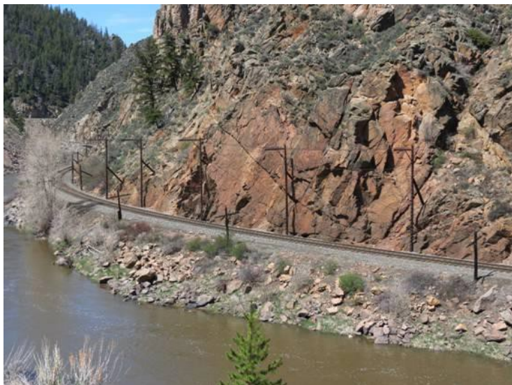
Figure 3.12. Rockfall Alarm Fence in Byers Canyon
